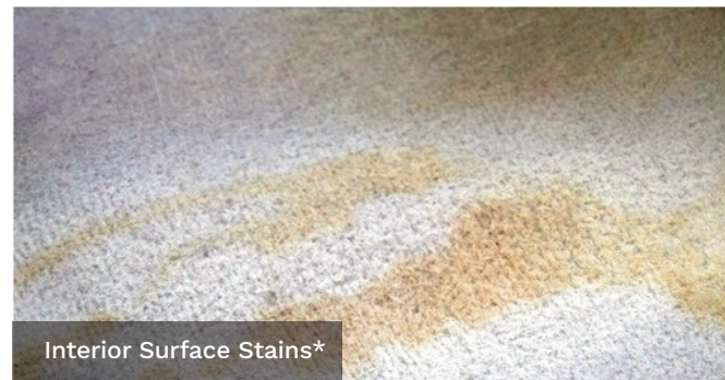
Bat Droppings Stains
